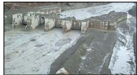
Chamoli: Damaged Dhauliganga hydropower project after a glacier broke off in Joshimath causing a massive flood in the Dhauliganga river, in Chamoli district of Uttarakhand. (PTI)
