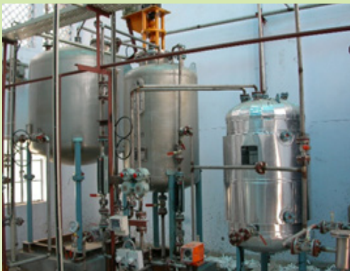
Explosive Processing Facility
