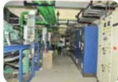
Compressors and PLC
