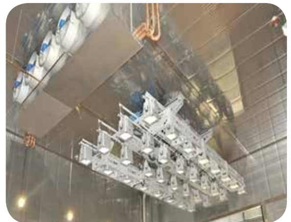
View of solar lamps and heat exchanger
